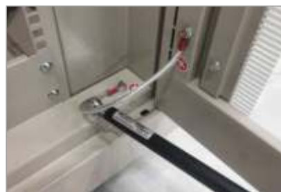
前、后门、侧板安装透明4mm 2 透明接地线 4mm 2 ground wire on front, rear door and side panel
